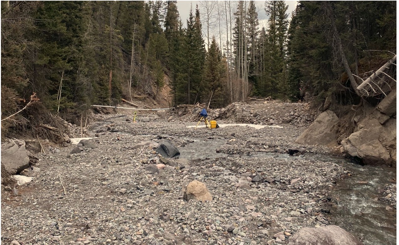
Figure 17 – Photograph is facing downstream toward the existing diversion channel on the right, showing the significant fill that must be cut to restore the channel.
