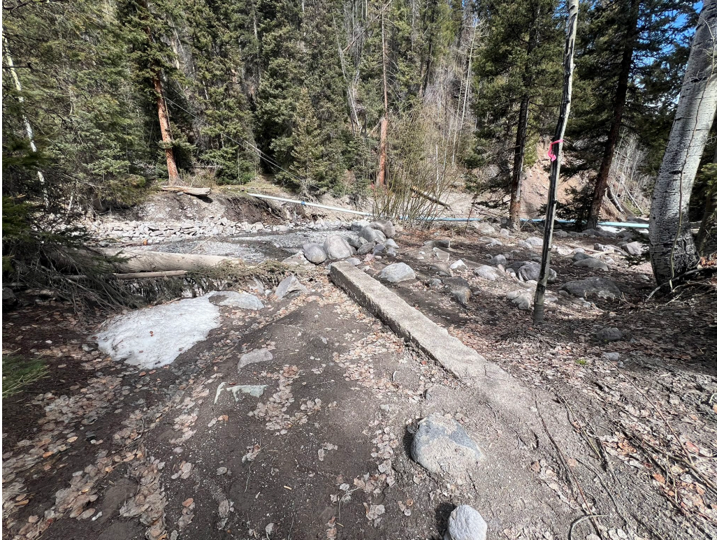
Figure 5 – Photograph showing the existing diversion structure filled with sediments. Only the top of the 4ft tall timber wall is exposed to the surface.
