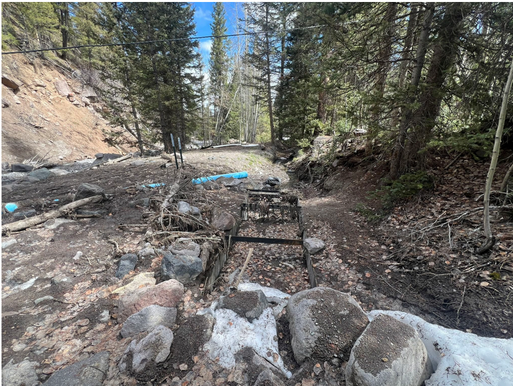
Figure 6 – Photograph showing the steel sediment channel and spring pipe. Notice the boulders that were transported and deposited at the head of the sluice channel.
